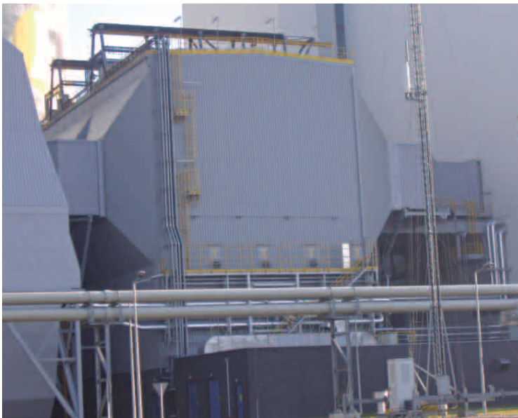
FIGURE 1: A recently commissioned Alstom electrostatic precipitator placed after an 850 MW lignite-fired boiler in Poland.
