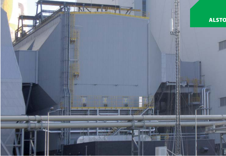
Figure 1. A recently commissioned Alstom electrostatic precipitator placed after an 850 MW lignite-fired boiler in Poland.
