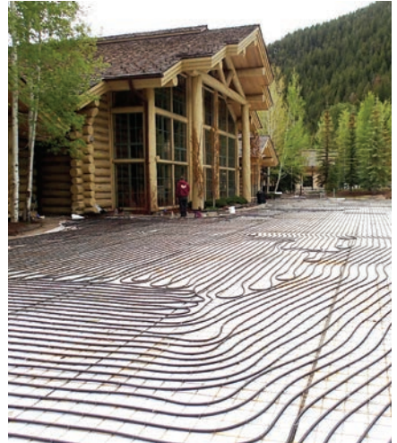
FIGURE 6. The tubing installed at Sun Valley Ski Resort in Idaho.
