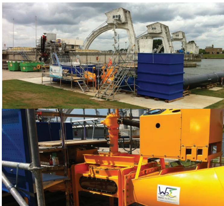
FIGURE 7 The Water2Energy water turbine prototype, about to undergo live testing.
